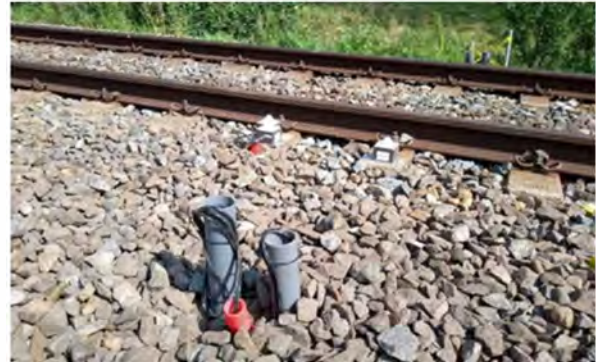
Two moisture sensors have been installed and are connected to the wireless sensor node via a cable
